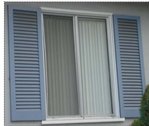
Below: This replacement aluminum sliding window does not give the same proportion to the facade as the original window.
