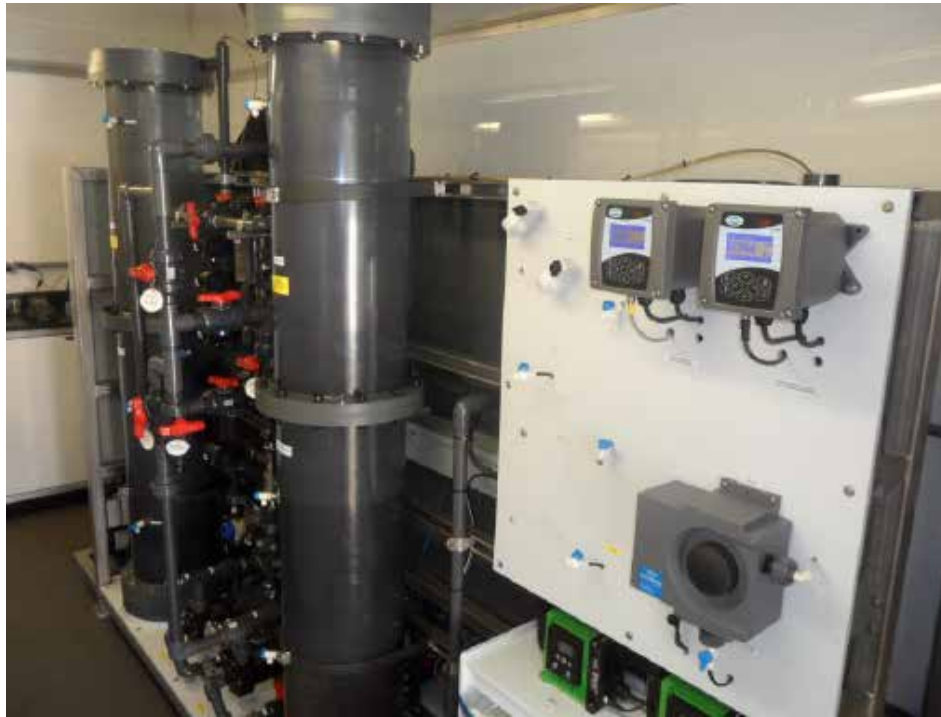
Figure 10 –Photograph of Cleanit® Pilot Unit
